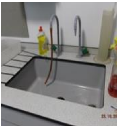
Figure 5: hose union taps are only permitted when backflow protection is in place (e.g. supplied from a storage cistern). The hose compromises the tap gap.
