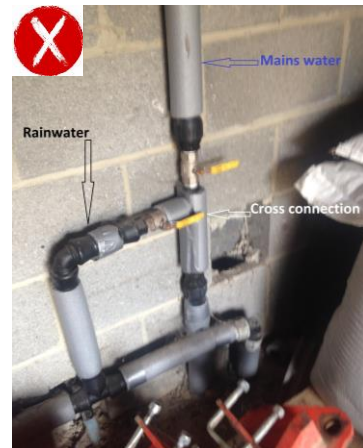
Fig 16: example of a cross connection between a rainwater and drinking water system
