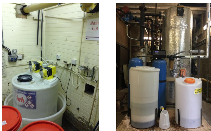
Fig 15: examples of equipment found in swimming pool plant rooms.
