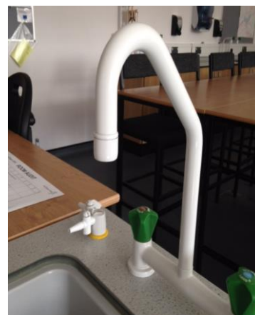
Figure 6: non concussive hose union taps (sometimes called hoseless taps) must be fitted in Fig 3: Scenario B – rooms 2, 3, &4. The tap gap must be maintained at all times
