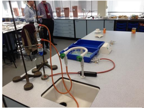
Fig 7: attaching laboratory equipment to lab tap compromises the "tap gap" – backflow protection is required e.g. supply from a storage cistern
