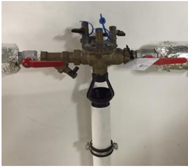
Fig 10: reduced pressure zone (RPZ) valve
