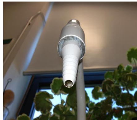
Fig 9: Any obstruction or interference with the air apertures, such as taping up or plugging, will eliminate the backflow protection placing the water supply at risk
