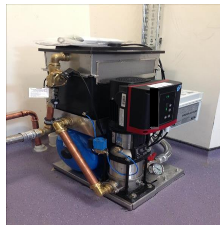
Fig 2: Storage cistern (break tank) supplying school laboratory
